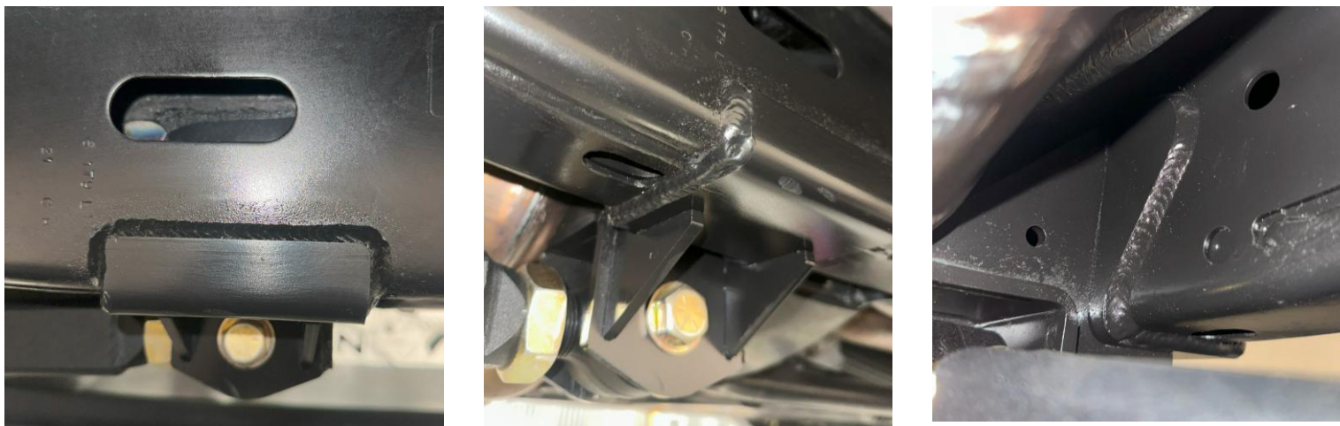
Figure 8: Bracket welded along edge to frame rail and area painted black
